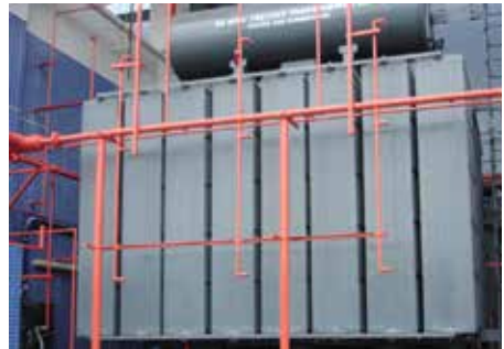
Image courtesy of CLP Power Hong Kong Limited
