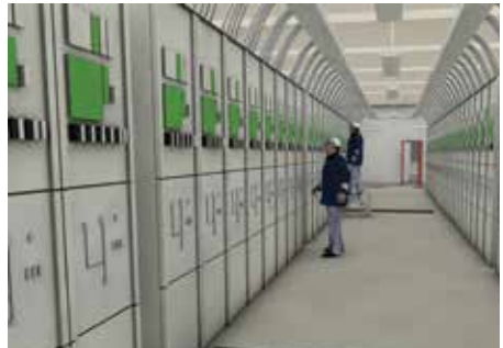
Image courtesy of CLP Power Hong Kong Limited
